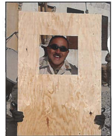
AFGHAN ALOHA -- Sgt. Kirk Halemano, from Kalihi, Hawaii, moves a door being fabricated for a motor pool at Kandahar Airfield, Afghanistan
